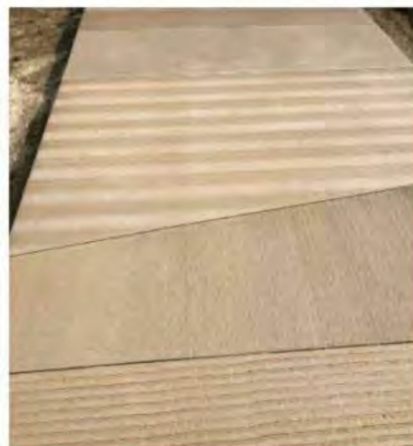
COMMUNITY CENTER PAVING - CONCRETE PAVING - FINISH: TOPCAST 01 WITH CUSTOM RAKED JOINTS - COLOR: SCOEFIELD CHROMIX INTEGRAL COLOR, COLOR TBD - 4" DEPTH WITH REBAR 18" OCEW
