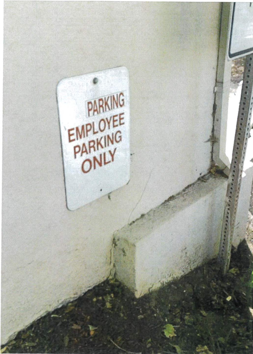
Photo 2 – Crack in Exterior Wall
