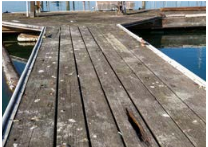
Deteriorated Marina Dock
