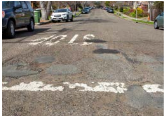
Street Pavement Damage
