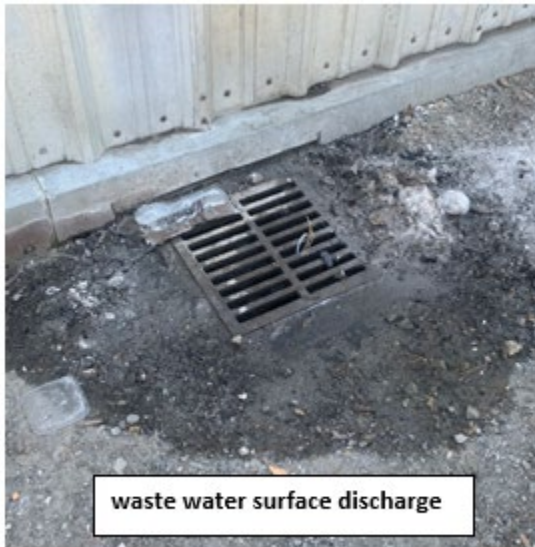
Imminent Health Hazard - Storm Drain
